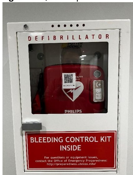
Figure 1: QR code placed on cabinet door.
